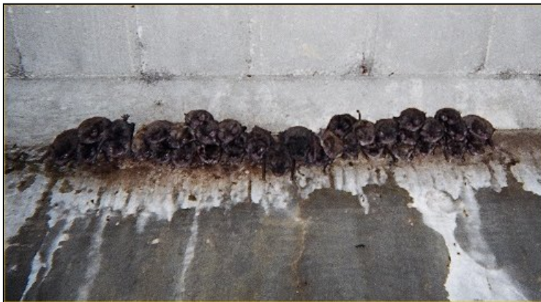
Photo 11: Bats Roosting & Associated Staining
