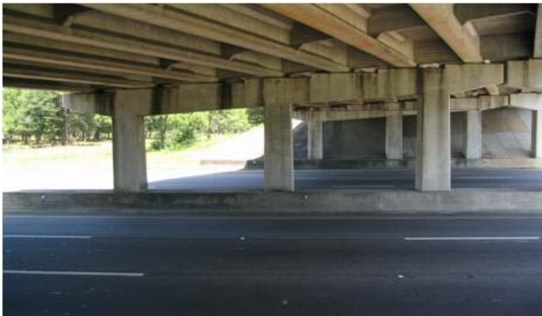
Photo 9: Staining on sides of pier caps
