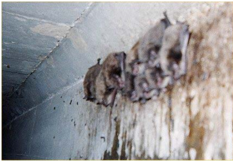
Photo 1: Bats hanging from cracks along Support beams
