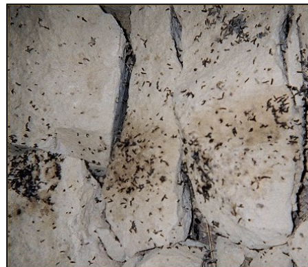
Photo 6: Bat Guano on Riprap
